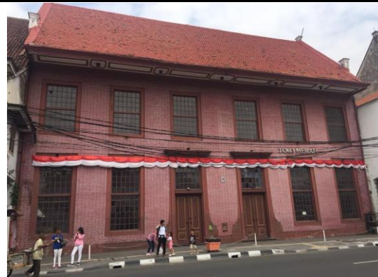
Source: Authors, 2019 Figure 3. Kota Tua Jakarta: Toko Merah or Red Shop, it is one of vacant building in Kota Tua Jakarta which becomes a rental exhibition space, and it is one of historical buildings
