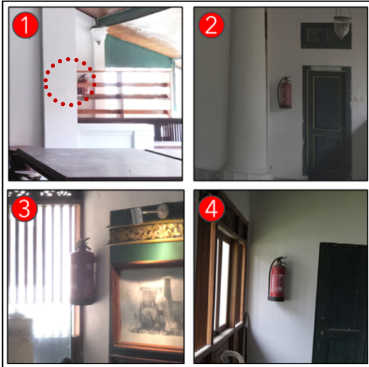
Figure 7. Photos of the existing fire extinguisher at R.A. Kartini Museum Rembang. (Source: Personal documentation, 2021)
