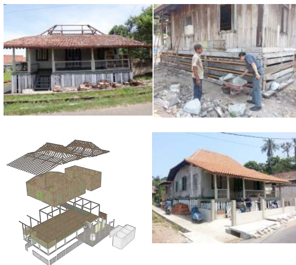
Figure 12. The demolition of the Malay Stage House, and the process for revitalisation in Kampung Tanjung (2015 - 2016), at 80% progress of adaptation in 2016. Source: Author.
