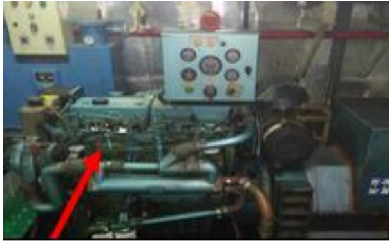
The engine driving the generator II
