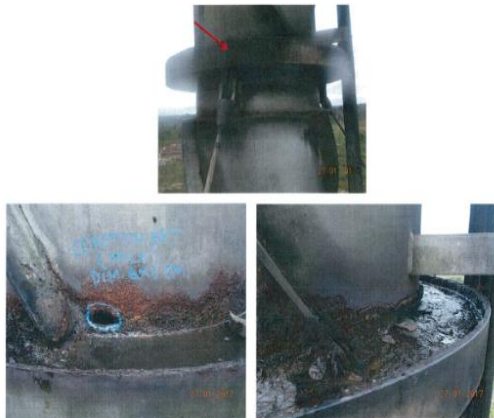
Figure 7. Hole Condition No. 1
