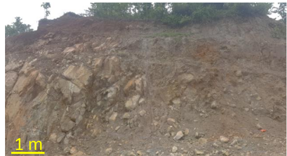
Figure 4. Slope conditions for scanline data in Region B140, with the yellow line indicating the length of the scanline.
