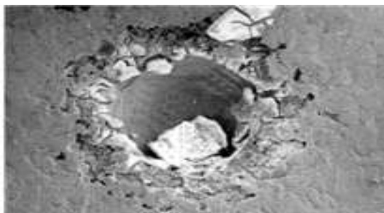
Gambar 5. Korosi Jenis Pitting Corrosion
