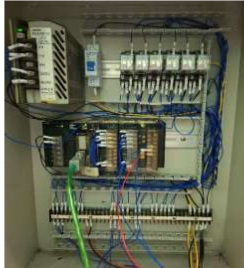
Gambar 5. Hasil wiring panel
