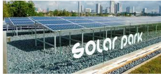
Gambar 6. Panel surya di Marina Barrage
