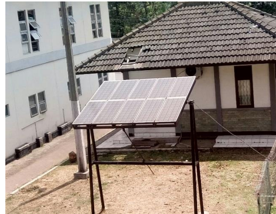
Figure 6. Tilt angle setting on PV plant
