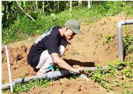
Figure 1. Squatting and stooping position in opening and closing ball valves activity
